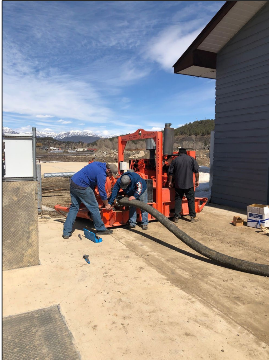
Staff Testing Diesel Bypass Pump at Pump Station One
